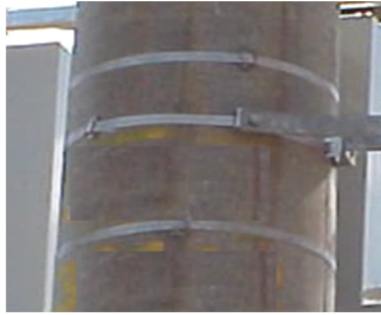
Figure 3: Typical stainless steel strapping used for installing communication equipment where drilling is not permitted.
