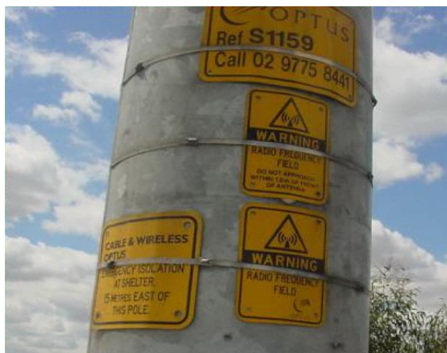
Figure 1: Typical safety signs placed on structures with communications transmitters attached
