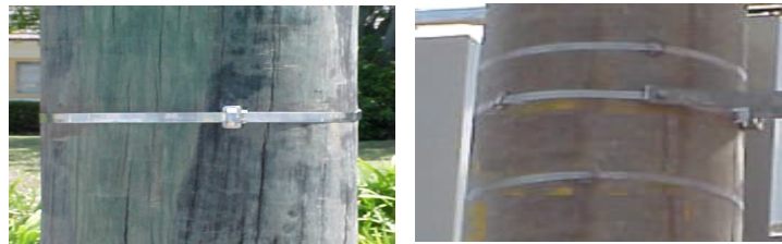
Figure 4: Typical stainless steel banding
