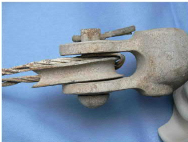
Figure 18: Incorrectly fitted helical termination
