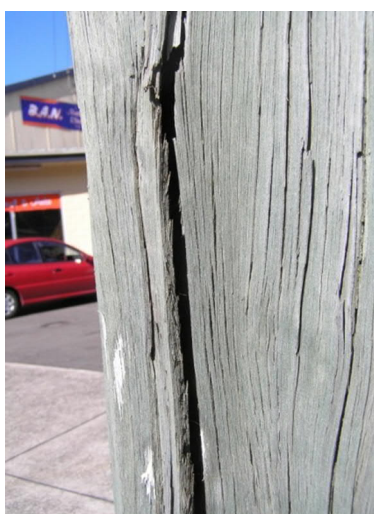
Figure 5: Loose sapwood on FPT pole
