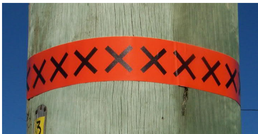
Figure 39: Condemned pole tape
