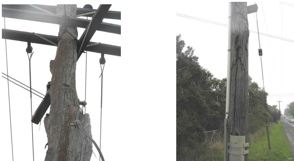
Figure 41: Example of poles considered for replacement due to the above ground condition
