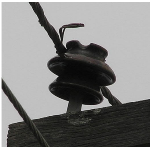
Figure 19: Broken HV tie wire
