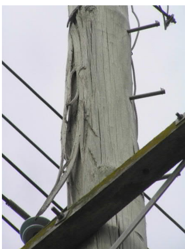
Figure 4: Loose sapwood on FPT pole
