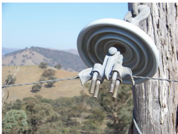
Figure 17: Missing nuts and washers on suspension clamp
