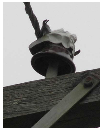
Figure 11: Damaged HV pin insulator (possibly caused by firearm) and broken tie wire
