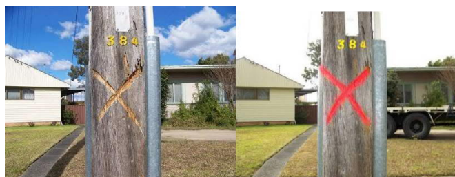
Figure 36: Marking of immediate priority condemned poles
