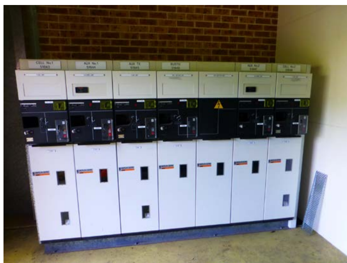
Fig. 5 Photo of installed SM6 switchgear
