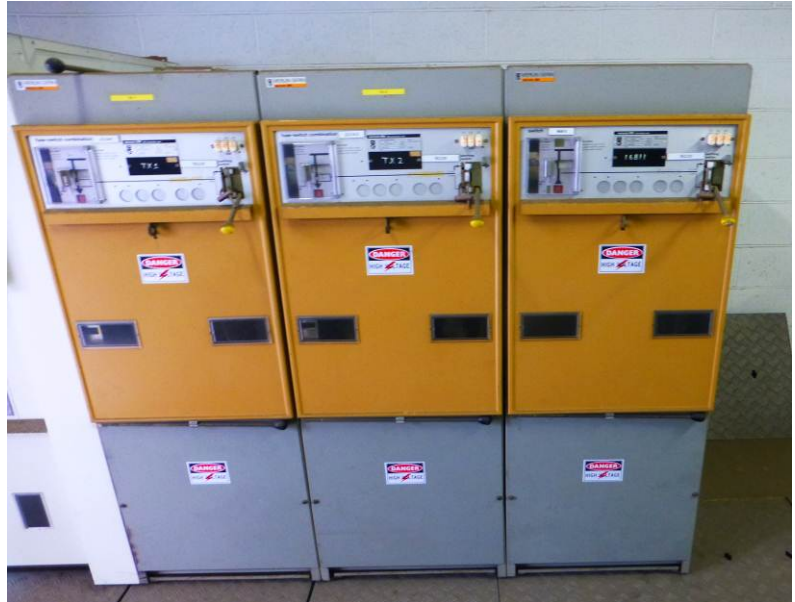
Figure 2 – Installed QM and IM unit
