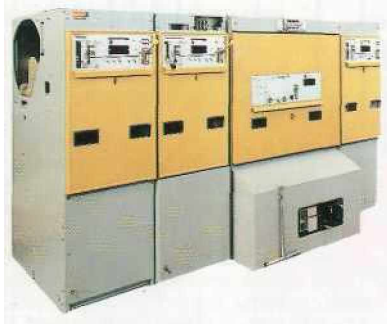
Substation with general protection and MV metering
