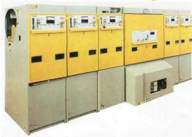
Substation with general protection and M.V. metering
