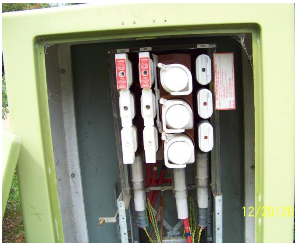
Figure 10 – An installed eSCI
