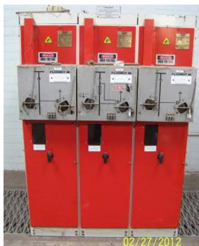
Figure 1: Installed IS/PFA/IS unit in an indoor substation
