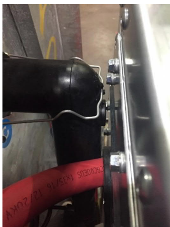
Figure 1: Pre-commissioned C-phase telcon termination with new clamp. Check for marks and damage and adequate separation prior to commissioning.
