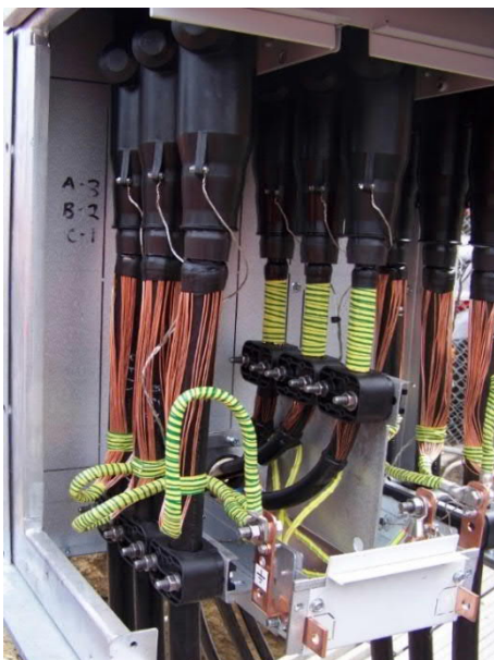
Figure 3: The completed terminations with the front and side termination cabinets panels removed to provide clear access.
