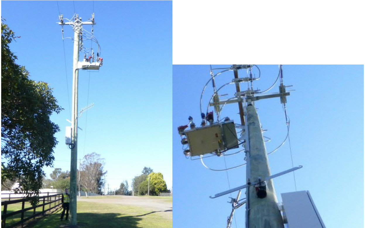
Figure 9: Photo of an installed recloser
