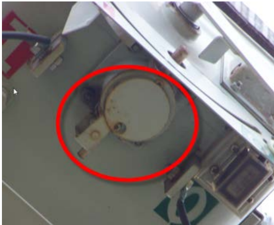
Figure 1 – Normal Iljin LBS condition (no defect)
