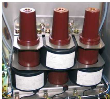
Toroidal-core current transformer on outer cone-type cable bushings
