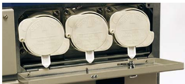
It is recommended that all three fuse links are replaced at the same time
