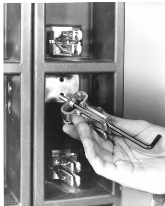
Remove top fuse contact from each phase to allow good access to busbar connections
