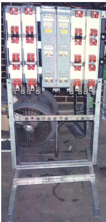
Distribution board with OEPS 800A isolator rather than the load break switch, and with fuse contact covers fitted.
