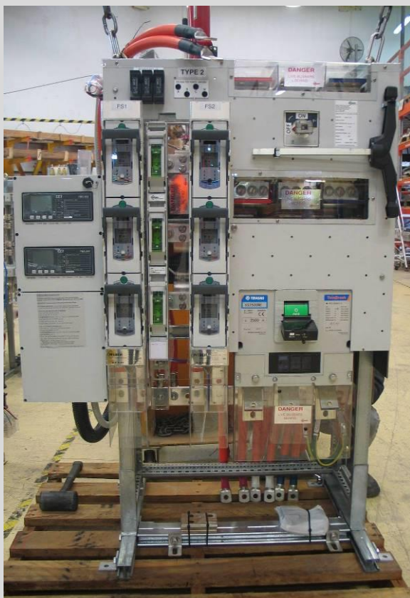
Type 2 – (Pre 2013) (Switch on incomer)
