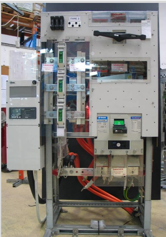
Type 3 – (Pre 2013) (Switch on incomer)
