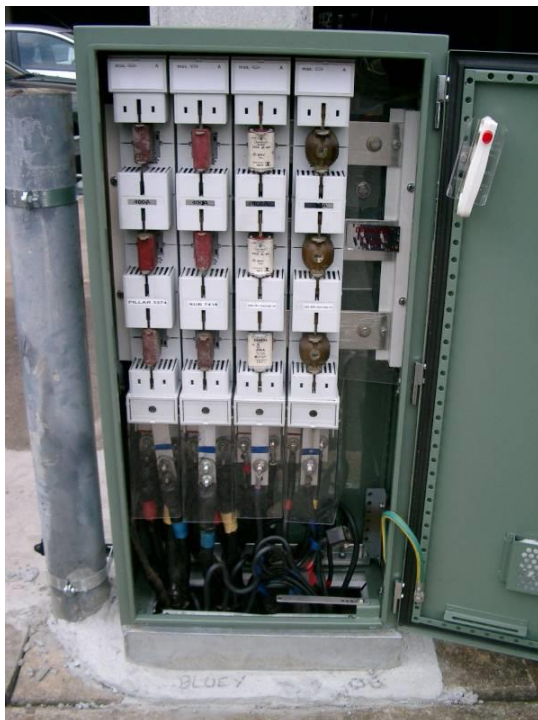
Figure 27: Example 5 - way cubicle (with older fuse strips)
