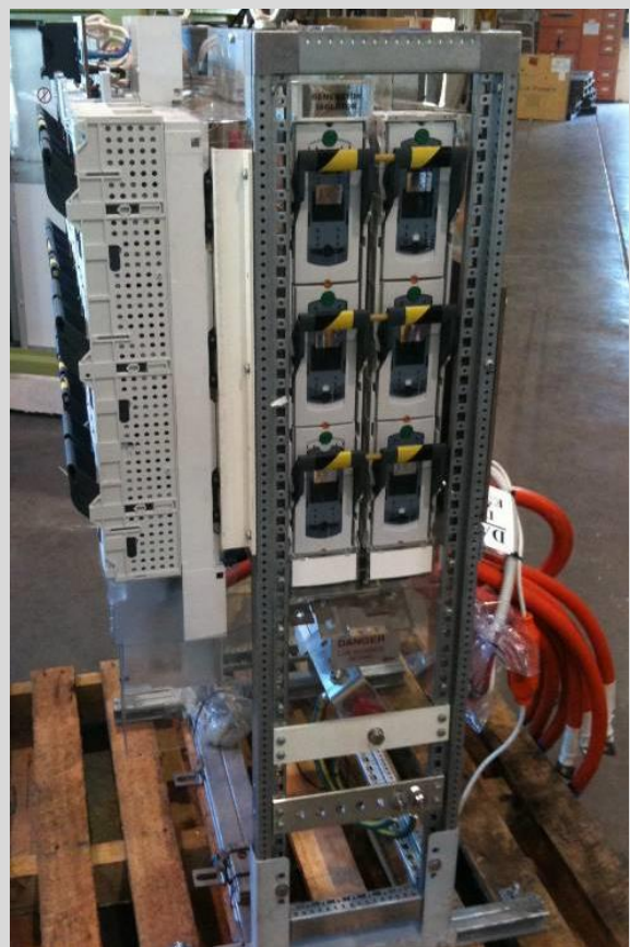
Side View– (2013) (Generator connections)
