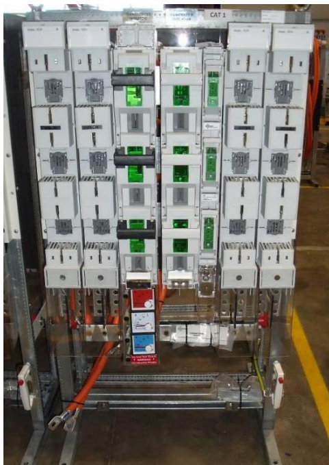
Cat 1 – (2006-2013) (No gap between fuse strips + new aux fuse)
