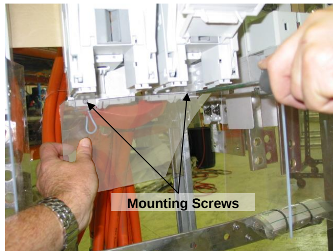
Figure 14: “C” phase transformer connection barrier
