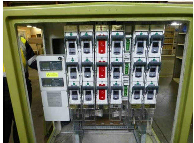
2013 Cat 1 LV board in a size 14 cubicle with MDI facing the end of the cubicle
