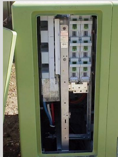
Side View– (2003-2006) (Generator connections)
