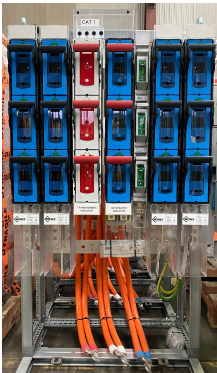
Cat 1 – (2013-Present) (No gap between fuse strips + aux fuse)
