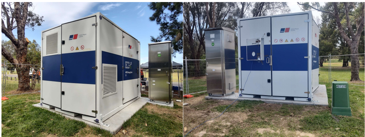
Figure 17: External earthing installation.
