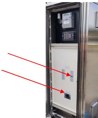
Figure 22: Electrical control panel.
