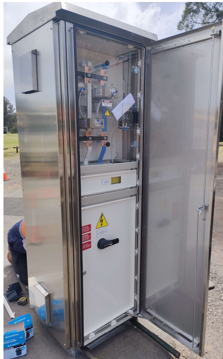
Figure 14: LV Switchboard opened for visual checking.
