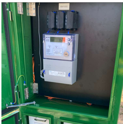
Figure 20: Metering with fuses
