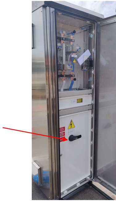
Figure 23: Location of main switch.
