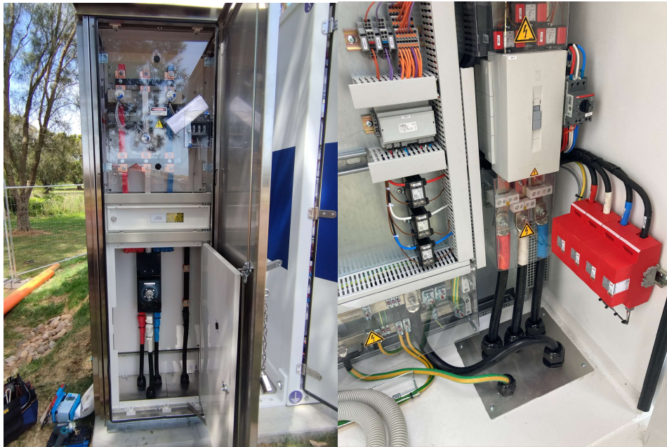
Figure 18: power cable connection between LV switchboard and BESS electrical area
