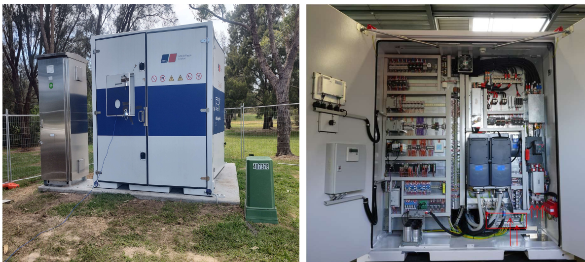
Figure 3: Image of installed Rolls Royce 'MTU' Energy Pack and electrical meter box.
