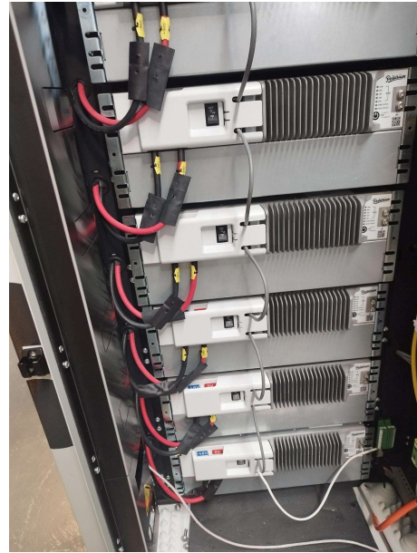
Figure 17: 3U battery installation.
