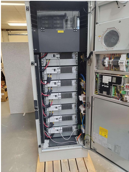
Figure 1: Typical Pixii PowerShaper battery unit with Polarium battery modules and inverters.
