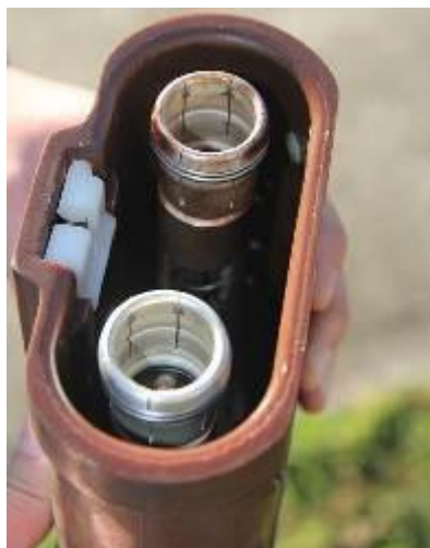
Figure 7-32: Discoloured main contact
