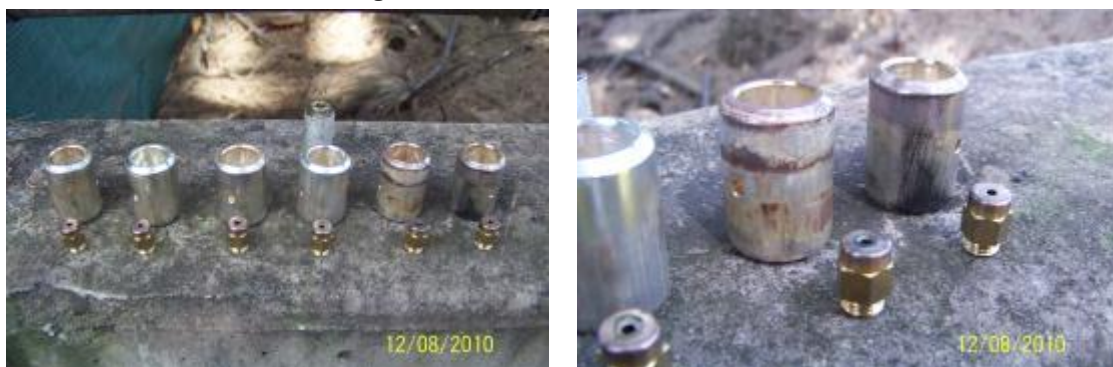
Figure 7-20: Damaged fixed main contacts
