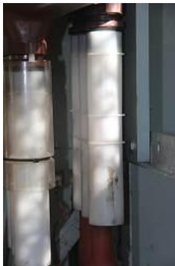
Figure 7-42: Dry termination with dust covers removed
