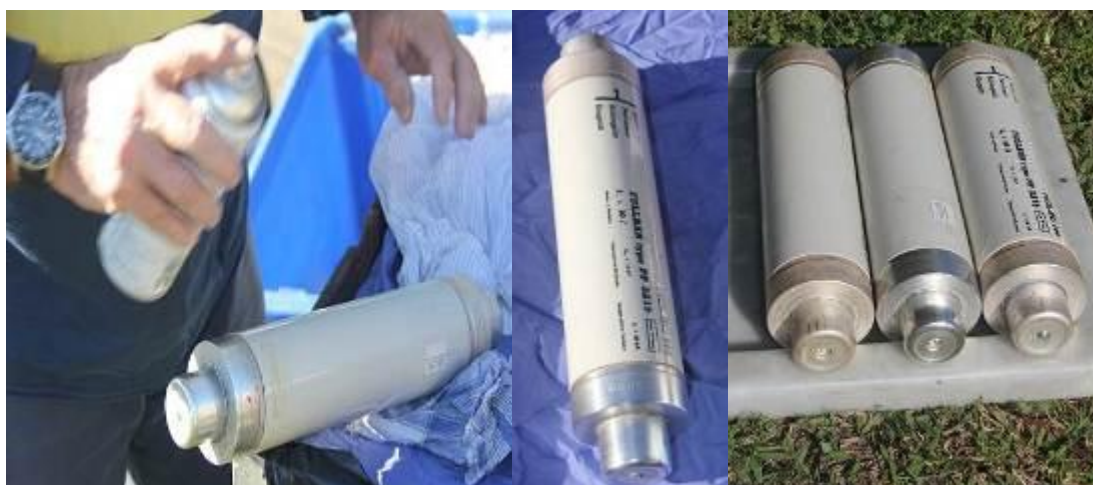
Figure 7-29: Applying contact cleaner and showing the final cleaned fuse
