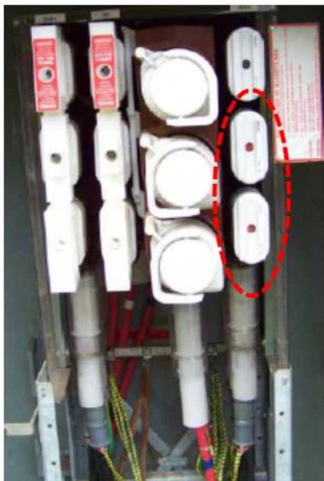
Figure 7-38: Switch caps indicating a fault
