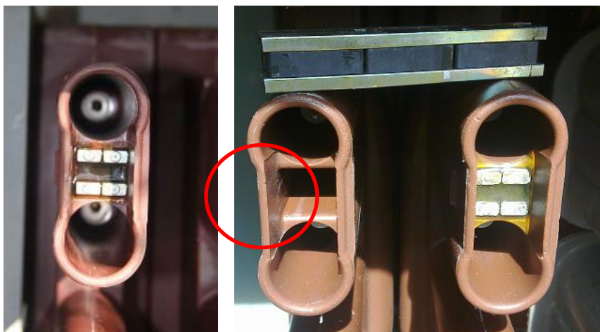
Figure 7-22: (a) Clean permanent magnet (b) missing permanent magnet
