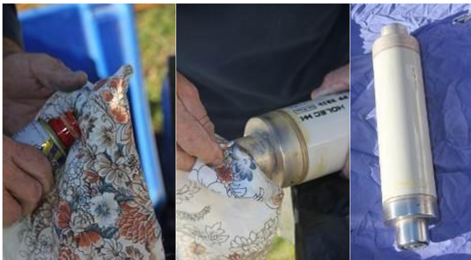
Figure 7-28: The use of Brasso to clean fuse contacts
