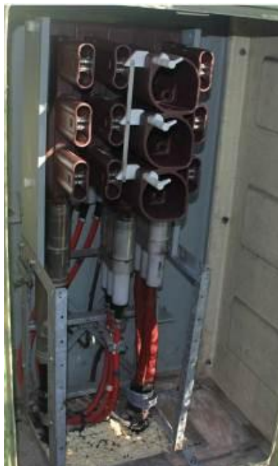
Figure 7-25: Switchgear after the cast resin has been treated
