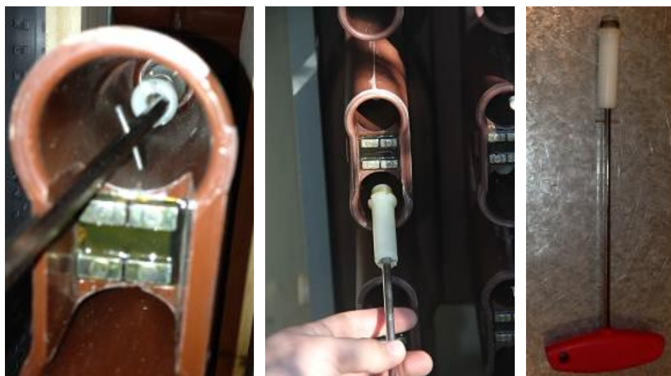
Figure 7-15: Removal of arcing chamber
